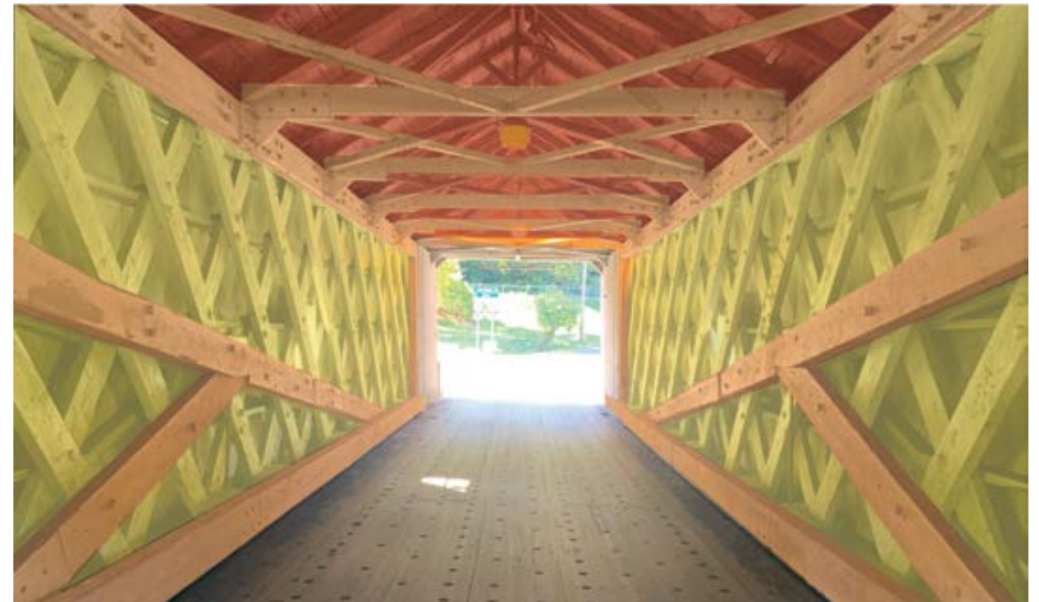
Figure 25: Re-designing how we define a new age of timber construction begins when we understand the full extents of Timber Construction in the present day, this early 1900's covered bridge displays multiple uses for Timber in one project. Early 20th Century Bridge. , Caruso, 2020
